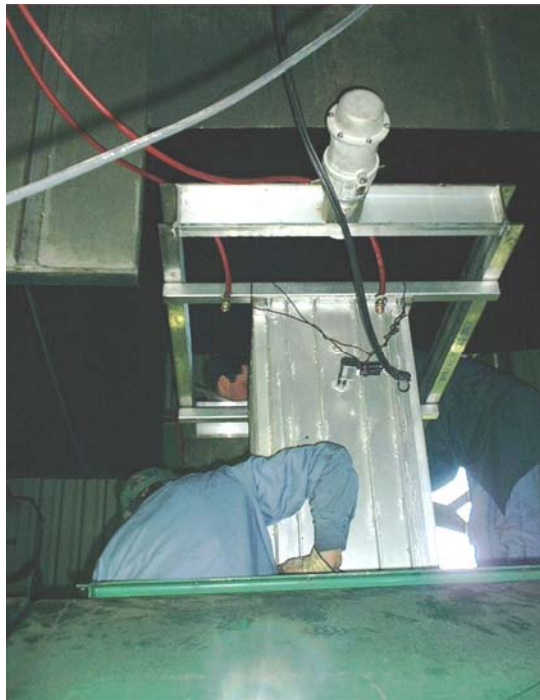
Figure 2. Exhaust Stack Extension and Sampling Systems
